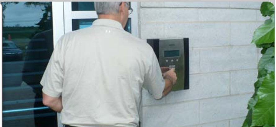
"Resident and visitor entry system"
